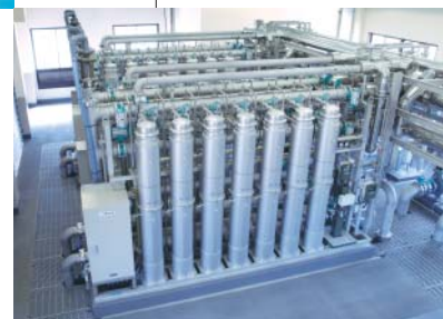
Membrane filtration units meet the requirements for a safe supply of water to the public.
